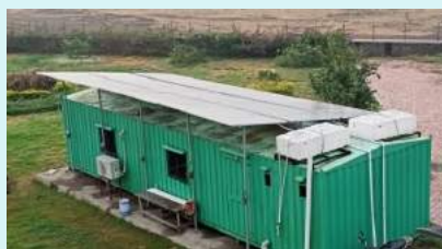
Solar power plant at Sinnar FSTP
