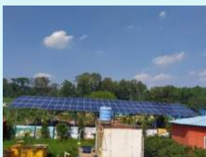
Solar power plant at Wai FSTP
