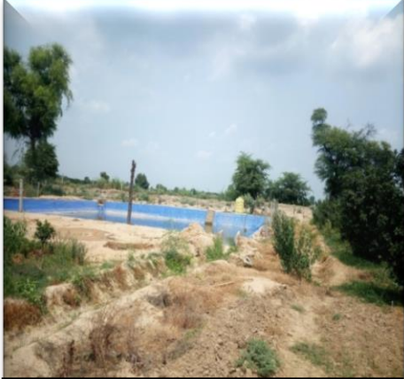
Farm pond constructed for storing water for Micro irrigation system in Abohar, Punjab
