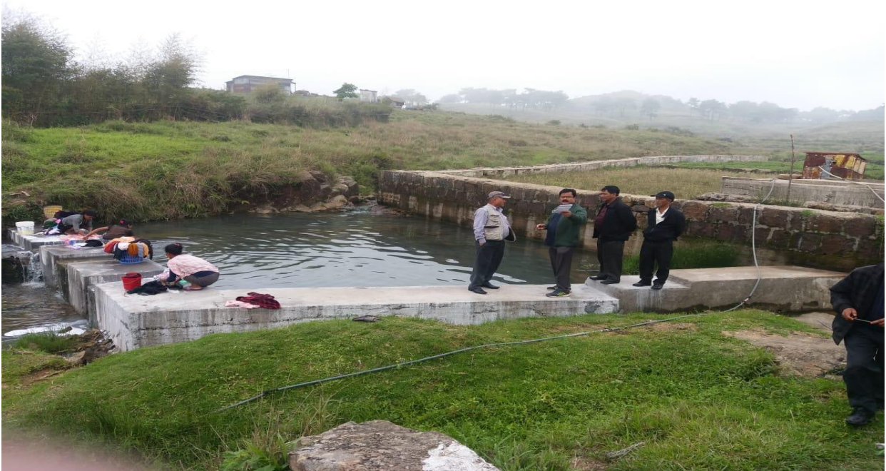
WAPCOS EXPERT VISIT CHECK DAM WASHIN PLATFORM WORK IN IWMP-V DISTRICT- EAST KHASI HILLS MEGHALYA
