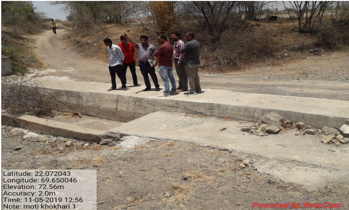
WAPCOS TEAM VISITED CAUSE WAY CUM CHECK DAM IN IWMP-II KHAMBALIYA JAMNAGAR
