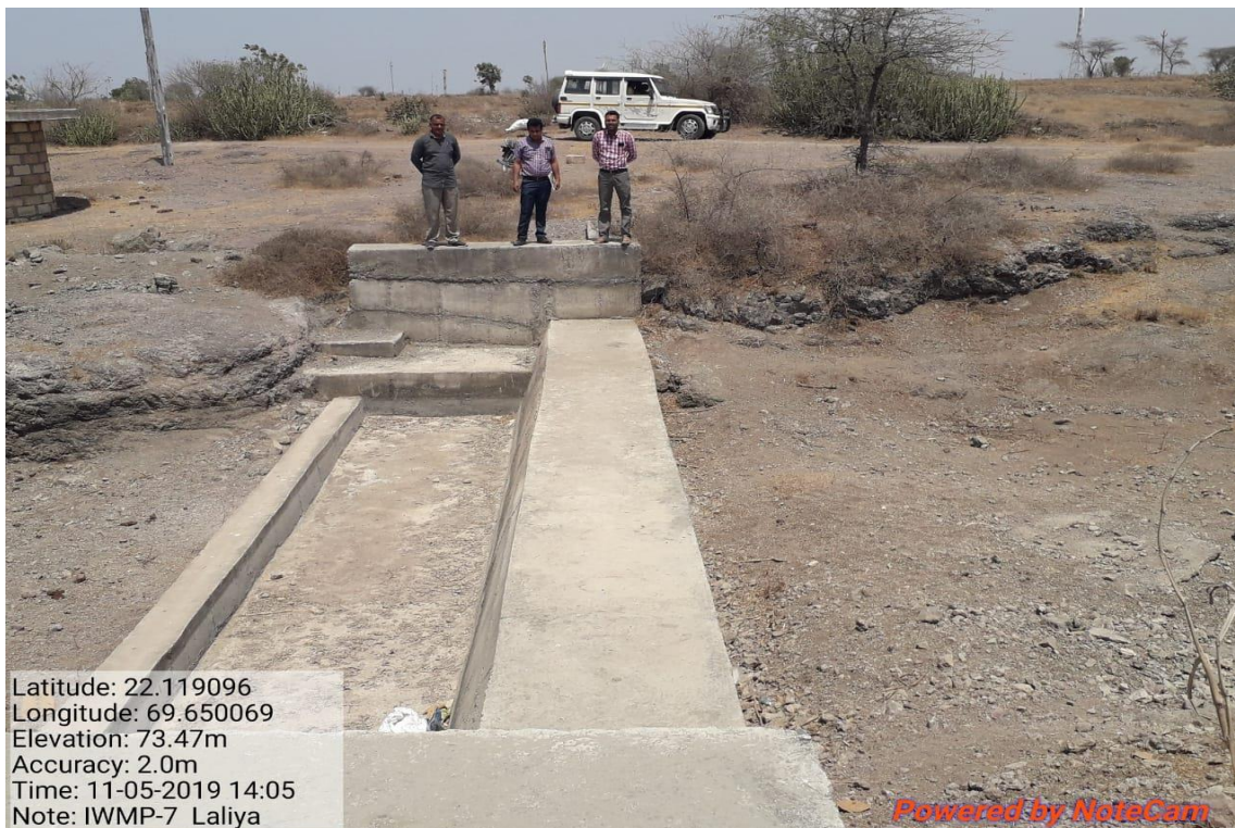
WAPCOS TEAM VISIT CHECK DAM IN IWMP-7 KHAMBALIA JAMNAGAR
