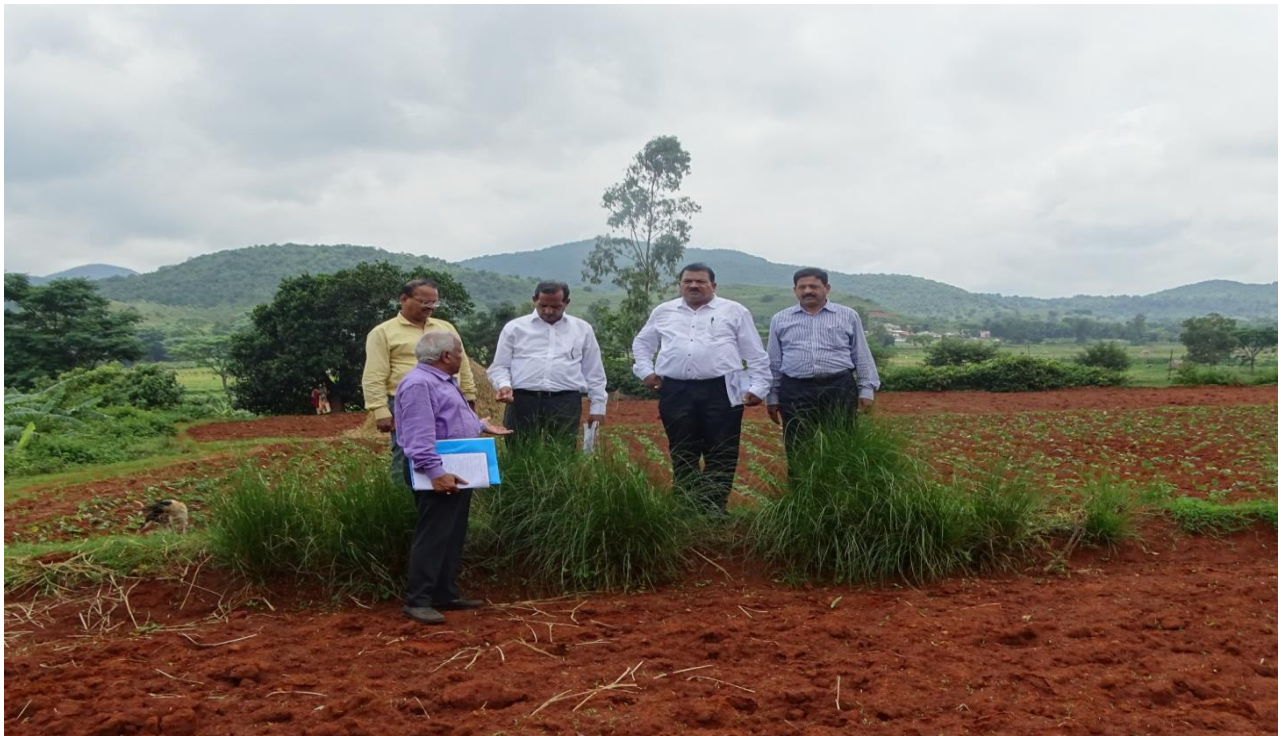
FIELD BUNDING AT VILLAGE- DUSURA, IWMP-V, BATCH-I, BLOCK- SEMILIGUDA, AREA- 4 HA, COST- 1.00 LAKHS
